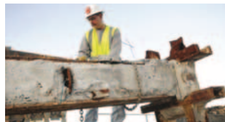
A workman from David H. Martin Excavating, Inc. wraps a chain around the beam before it is offloaded near the construction site at the PSC on Industrial Highway next to the Harrisburg Campus.
